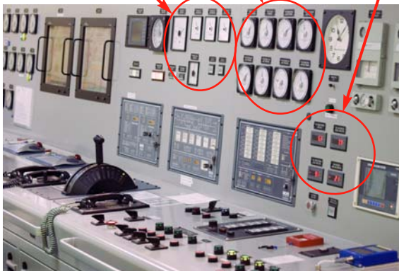
Bridge and flying bridge control panels
