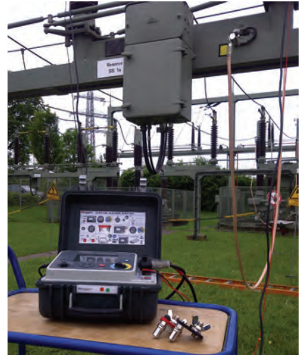
DLRO100 testing circuit breaker
