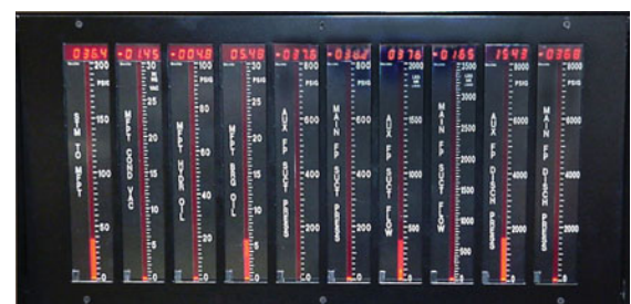
Bargraph Draft Gauges in Rack Panel ▲
